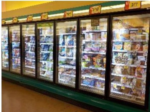
Pulsing doors on low temperature cases for supermarket chain.
