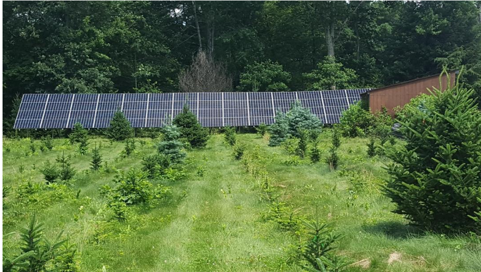
Figure 5: Ground Mount Solar System at Bedrock Tree Farm, Wakefield, RI. This array offsets 100% of electricity usage, with a payback period of only 3-4 years. Three different programs were used for the funding of this project: RIAGEP, REAP, and the Renewable Energy Fund.
