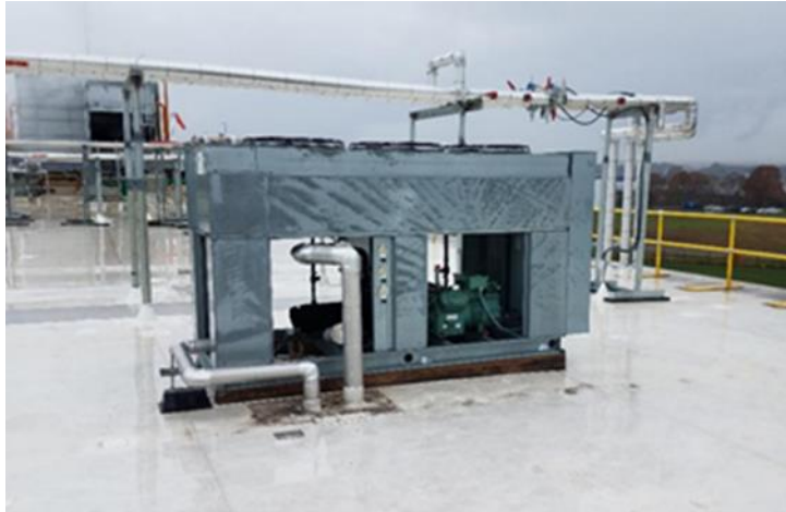
Rooftop condenser and compressors packaged in one unit at the customer's site in North Kingstown, RI
