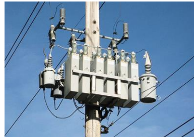
Power Factor Correction with Utility Capacitor Banks
