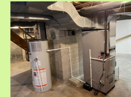
HEAT PUMP WATER HEATER
