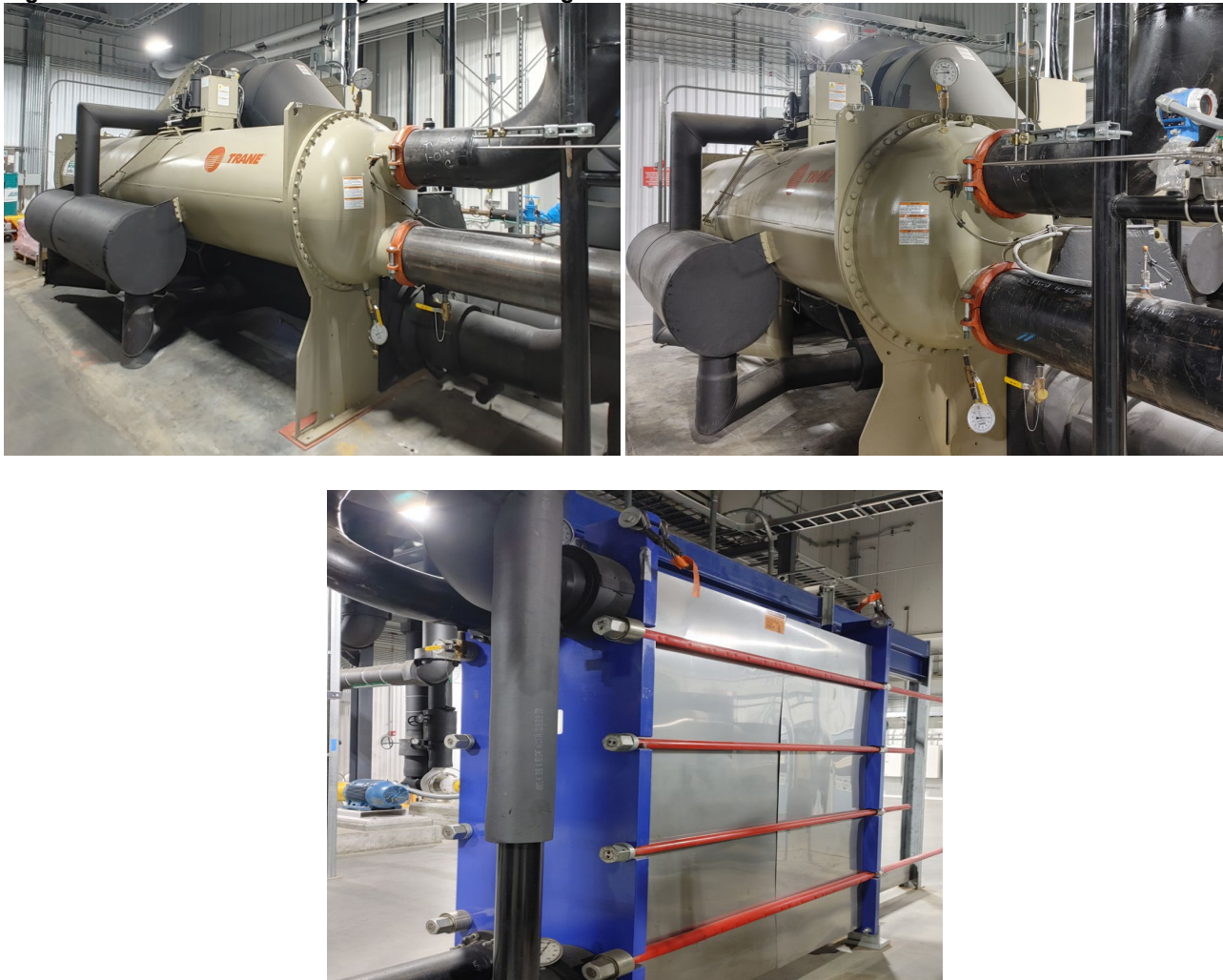
Figure 2-14 Chillers 1 and 2 along with heat exchanger
