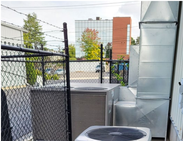
Photo 2-7. 12.5-ton packaged HVAC unit nameplate
