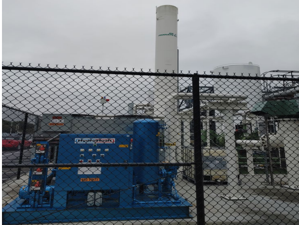
Figure 2-13 New Cryogenic Nitrogen Generation plant
