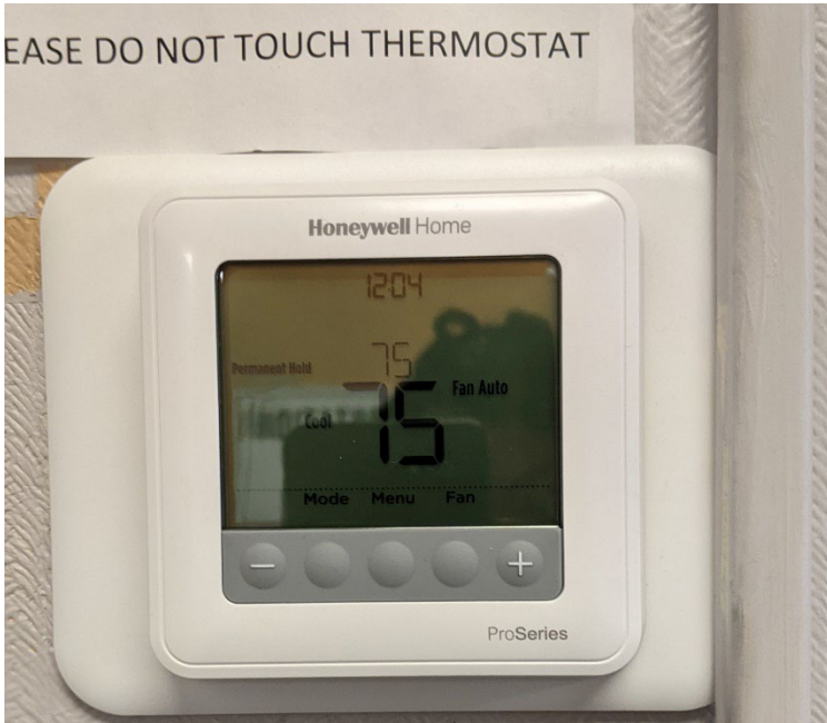
Figure 1-5. Zone 4 transportation office non-smart thermostat
