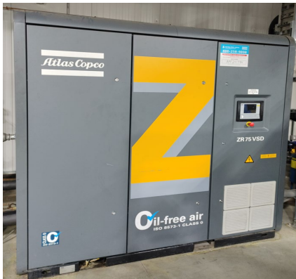
Figure 2-12 New 100 HP VFD Compressor
