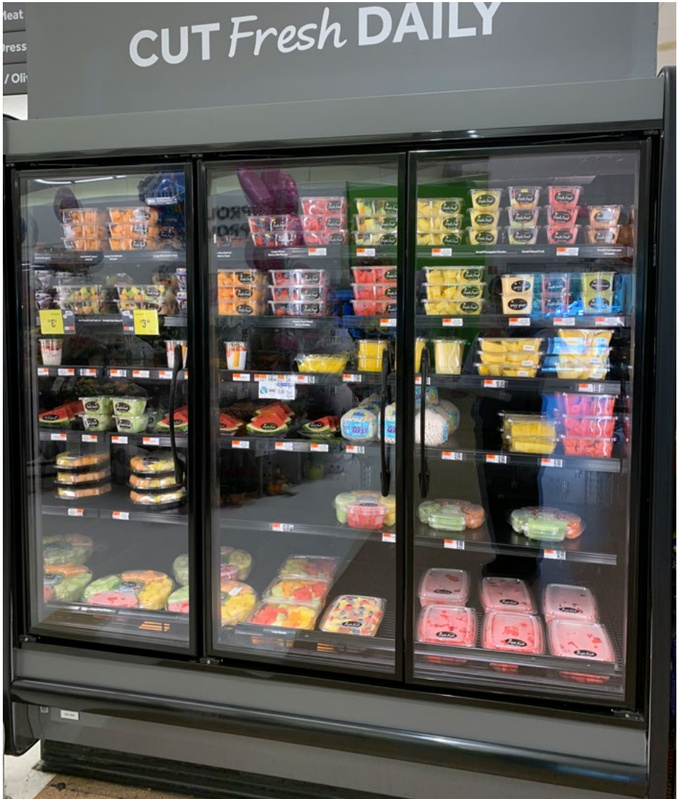
Figure 2-2. Example of installed doors on a refrigerated case serving fruit
