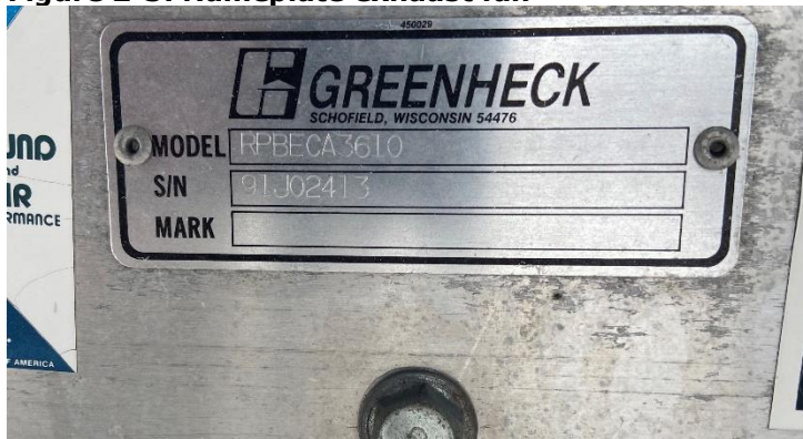
Figure 2-3: Nameplate exhaust fan
