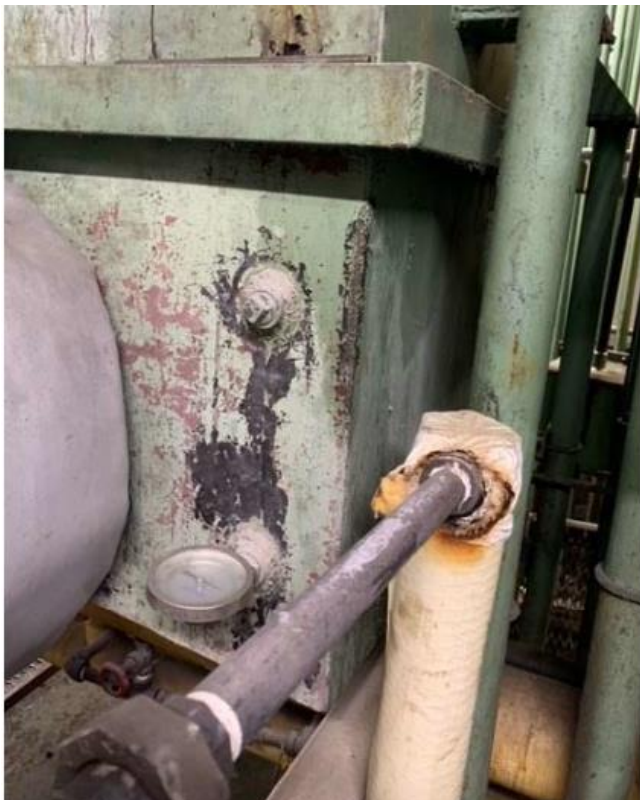
Figure 2-12. Steam or condensate line existing insulation
